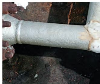
Corrosion Under Insulation
